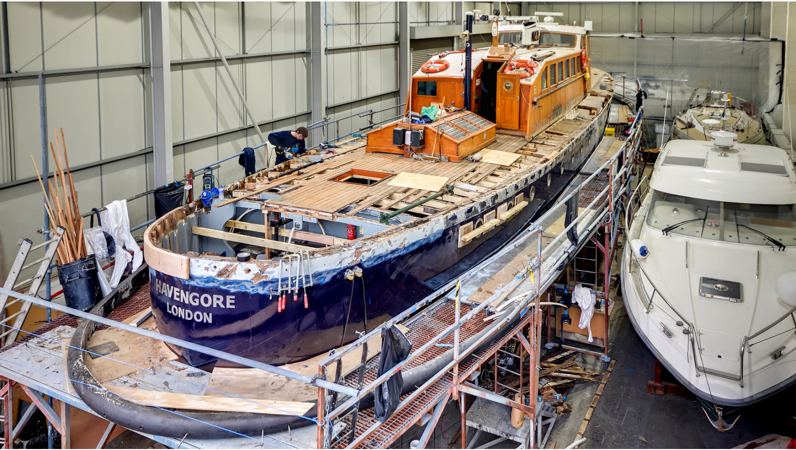
MV Havengore Undergoing Extensive Restoration to its Decks and Associated Structure at Fox's Marina and Boatyard in Ipswich
